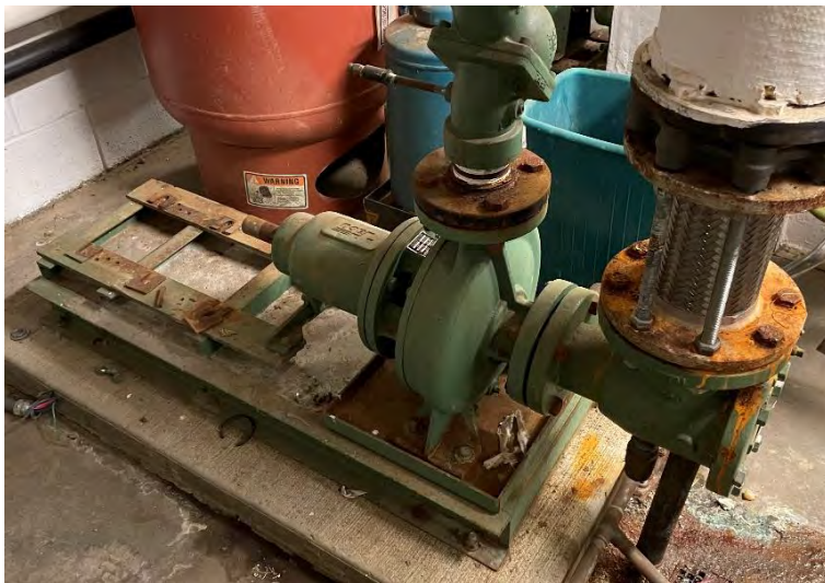
Photo 3: Heating Hot Water Pump Without Motor
