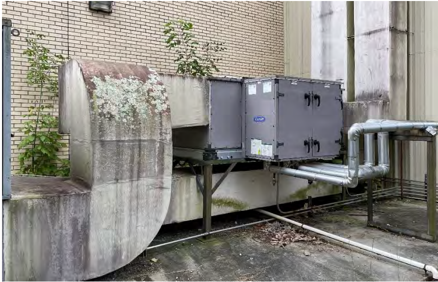
Photo 6: Cell/Housing AHU and ERV
