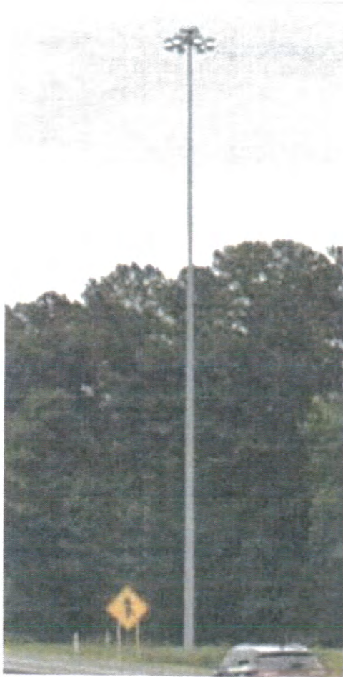
High Mast Lighting – Daytime Source: Anderson County
