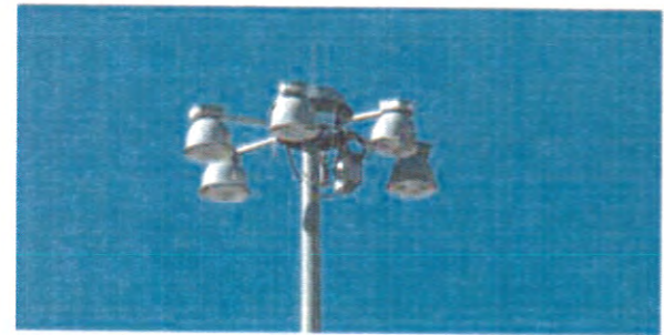
High Mast Lighting – Fixture Source: Singh & Associates
